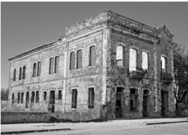
Figure 8 Explosion Shocked Building
